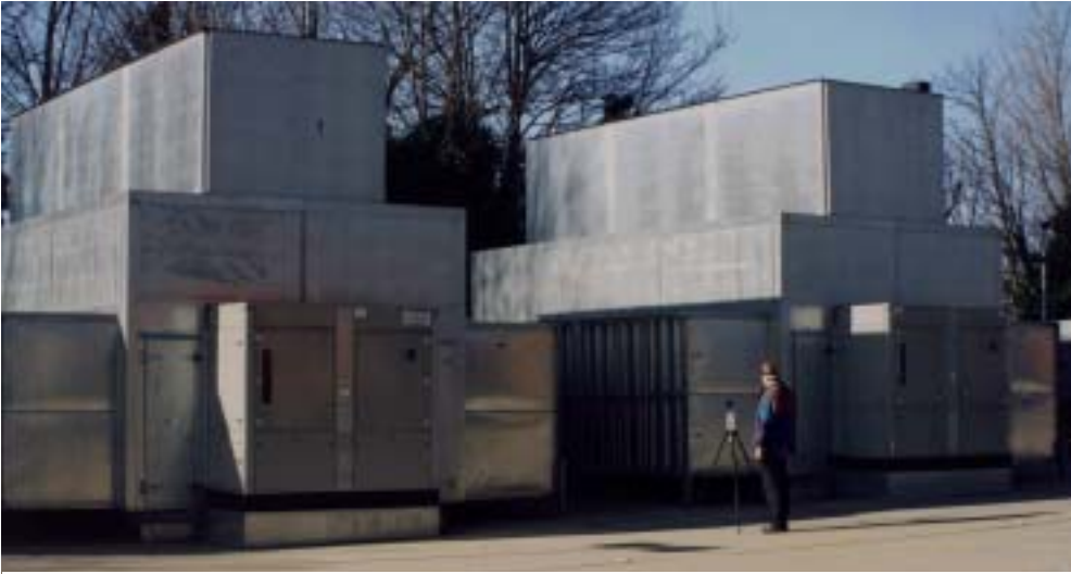
Photograph showing two air-cooled water chillers with full attenuation packages.
